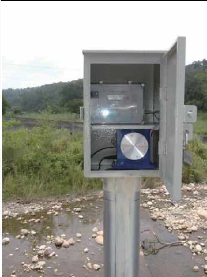
TW-264S connected to Level Logger, Battery powered.
