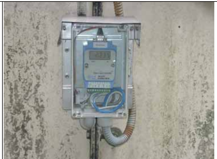
Display and transmitter for TW-265S on sidewall of tank
