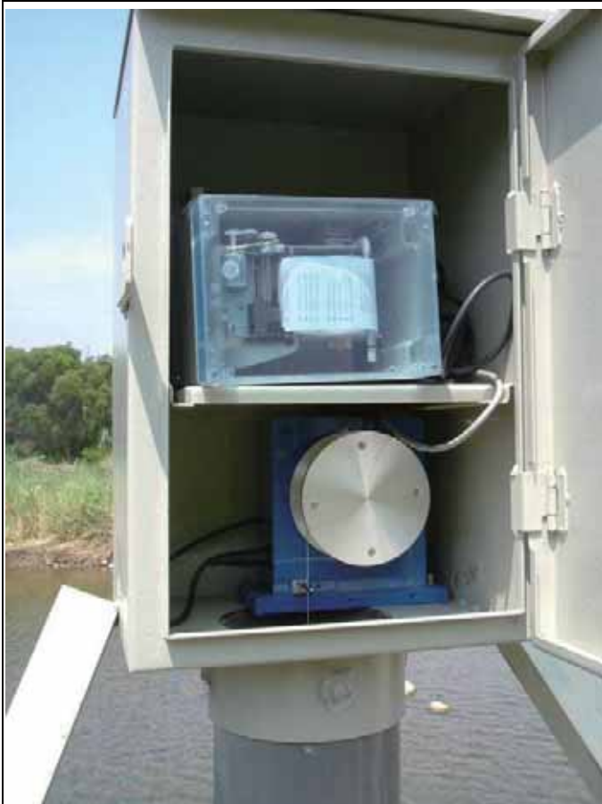
TW-264S connected to Level Logger with typing recorder
