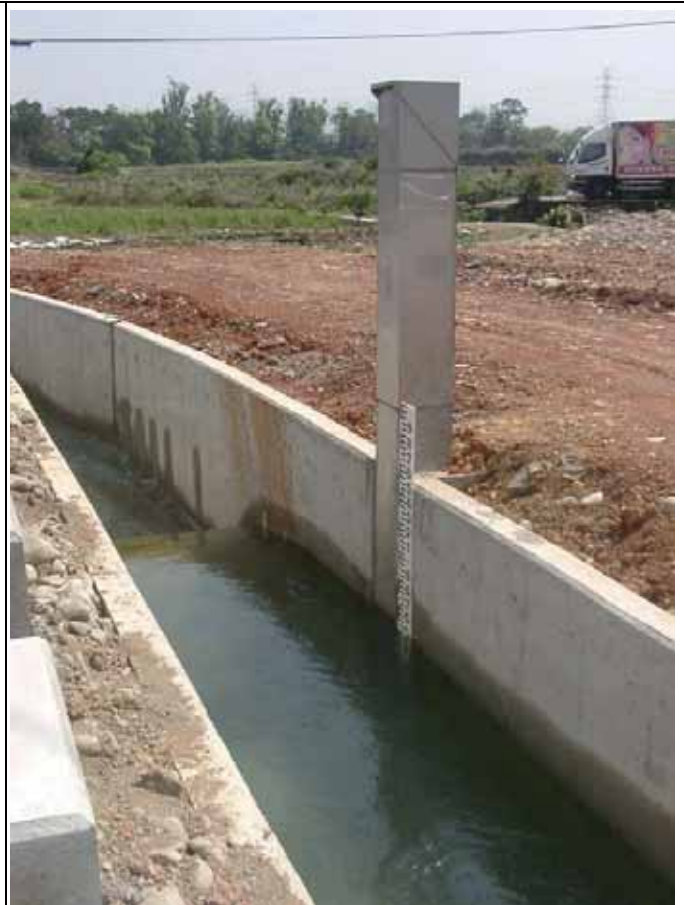
Level monitoring for long-throated flume in a U canal.
