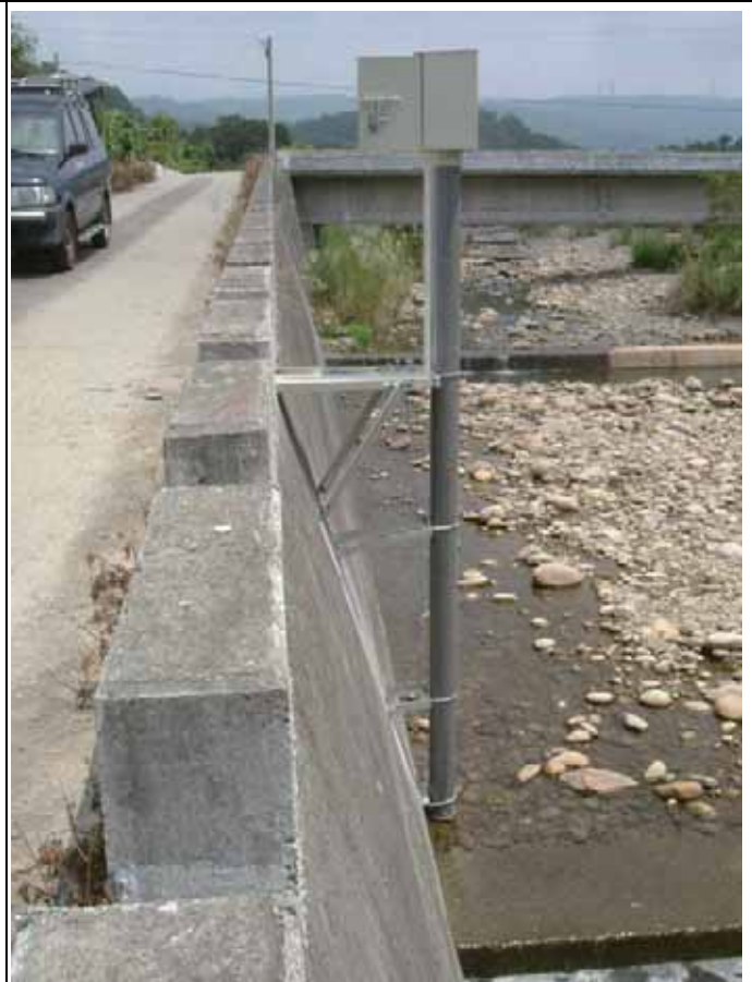
Float-Operated Level Station in 6" Still Well.
